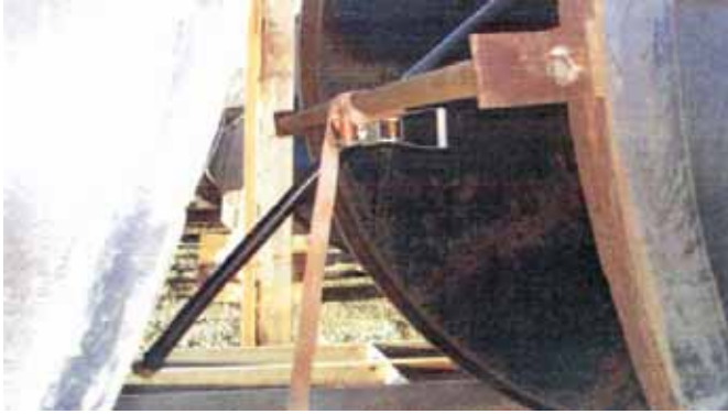
How the pipe was secured on the reel using a ratchet strap.
