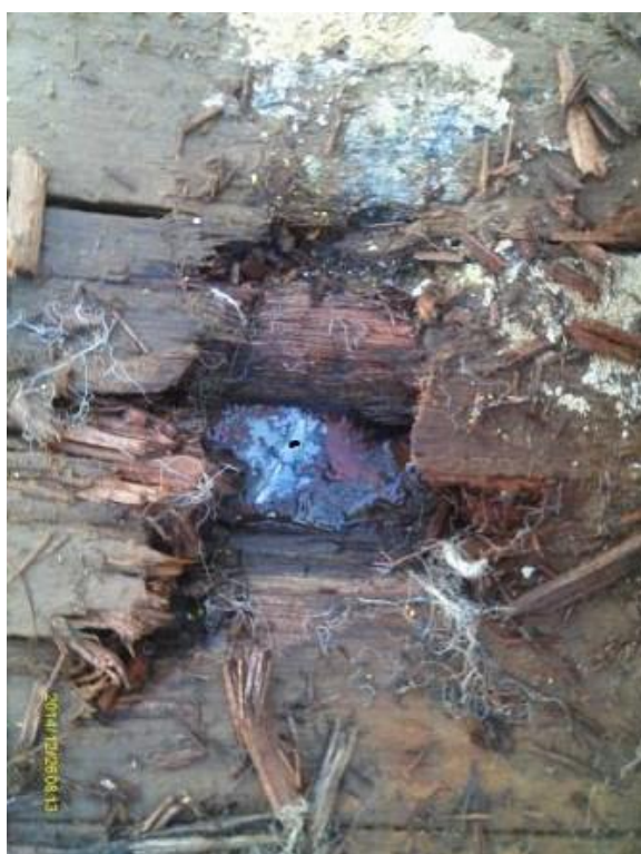
Figure: showing damage to deck
