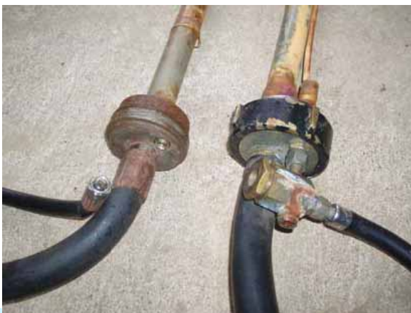
Damaged safety relief valve assembly
