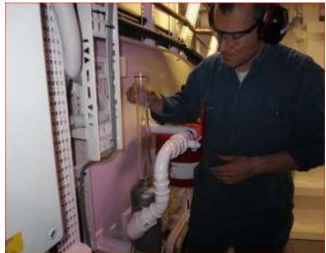
Emitter protection tube lowered into the filter (picture from another vessel).
