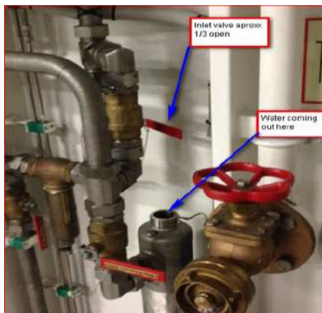
Investigations revealed the inlet valve was approximately 1/3 open
