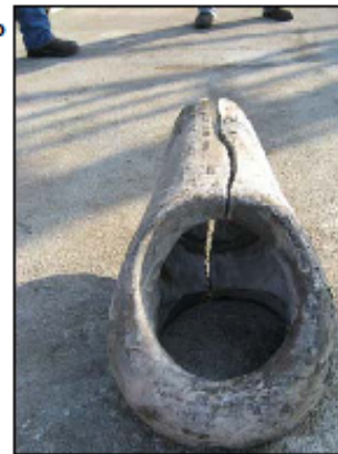
Failed Mooring Socket
