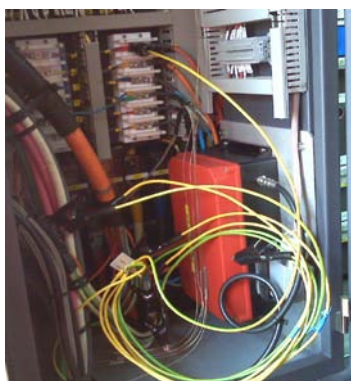
High voltage (HV) junction box with earthing equipment attached
