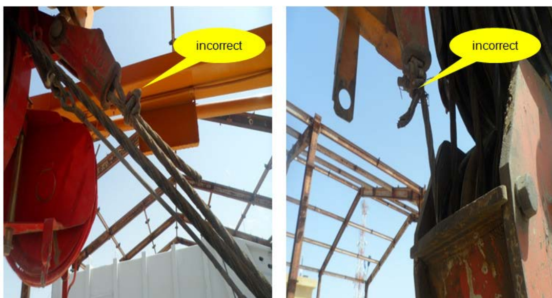
Figure: Showing incorrect fitting of wire rope grips
