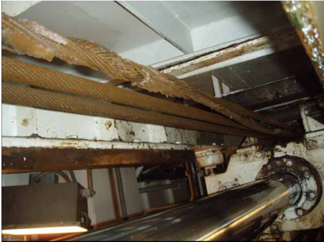
Photograph showing partly parted wire
