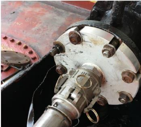
Bunker hose connection at ship's bunker manifold
