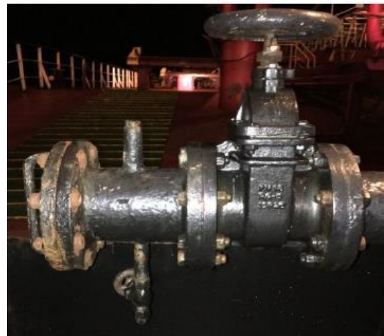
Ship's bunker manifold valve
