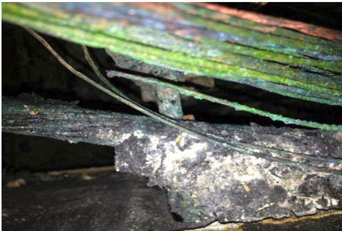
Figure 1: Generator cable caught fire suspected worn wiring over time and lay out cables over the terminal
