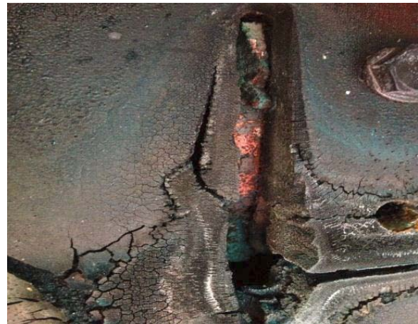
Figure 2: Phase 2 of the generator bus bar possibly contacting the generator casing; thus burning through phase 2 bus bar
