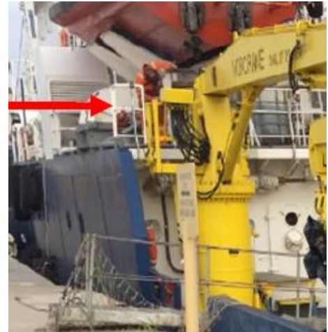
Arrow showing welder working with unprotected edge behind and potential to fall into water
