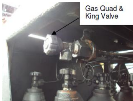
Gas quad and King Valve
