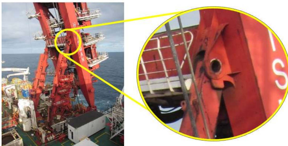
Right: Close-up of the adjuster leg housing (with bolts, keeper plate and pin missing)
