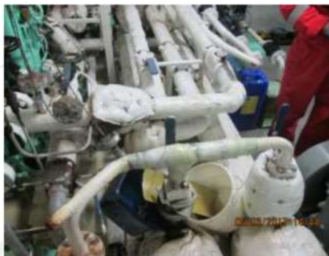
Complex shape and fitting of pipe
