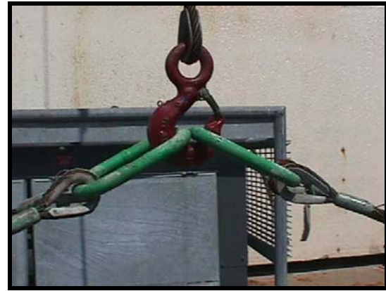
Figure 2: Similar hook point with incorrect sling angle=hazard.
