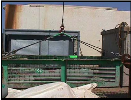
Figure 1: Similar cargo basket with incorrect sling angle.
