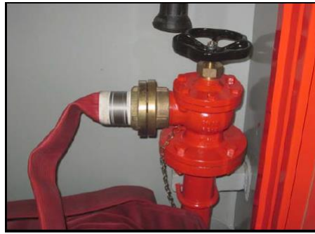
Fire hydrant with correct 65mm coupling (compatible with 65mm hose coupling)
