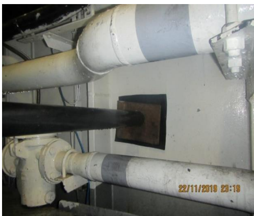
Water ingress temporary repair
