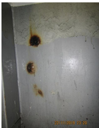
Showing condition of sea chest
