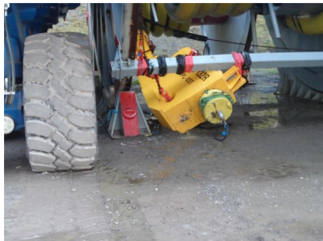
Figure: showing cradle and damaged pullhead
