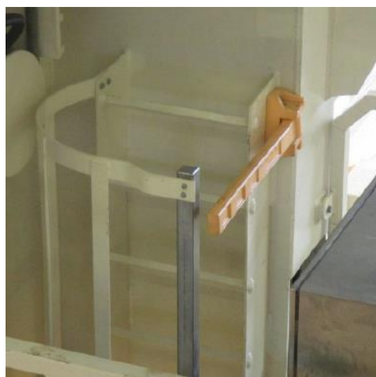
Figure: ROV LARS ladder guard (plastic) reinstated
