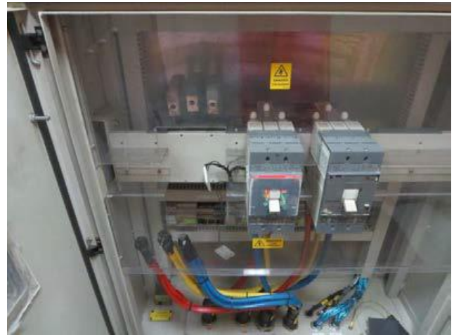
Figure: uninsulated wire terminals
