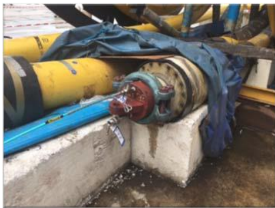
Showing 6" pull head that was removed for inspection of the foam pig
