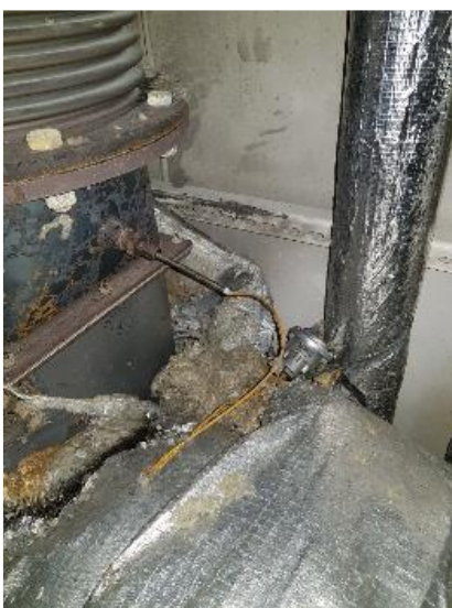
Exhaust sensor was tampered with
