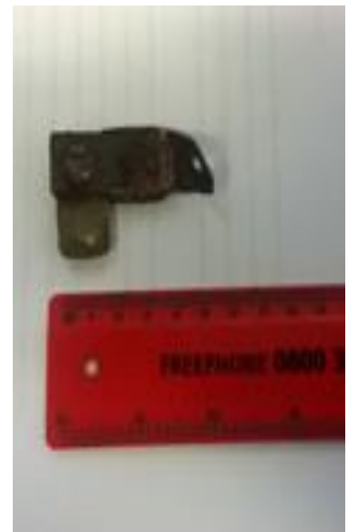
One of the rusted fastening brackets
