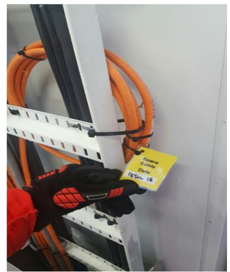
Properly tagged cable
