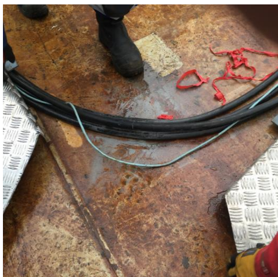
Cables routed across the deck
