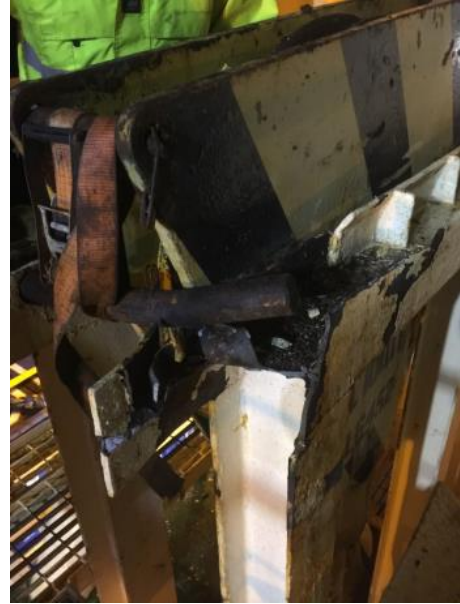
Section of H-beam (post collision with headache ball and hook)
