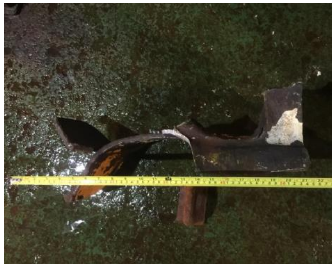
Section of damaged H-beam
