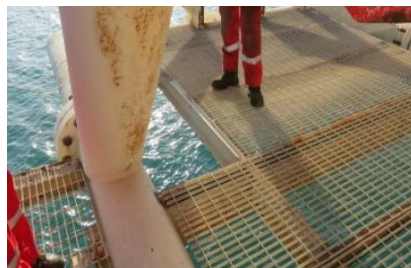
Opening through which person fell
