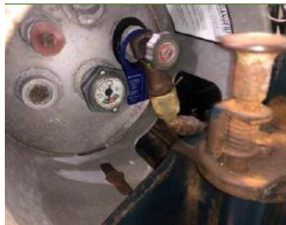
Tank valve and fuel line
