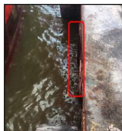
Missing fendering at berth
