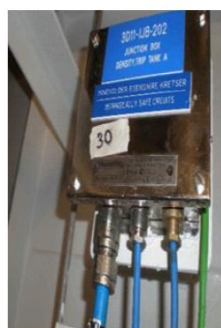
Improper Cable Gland Installation/Modification
