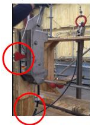
Image 1: The release handle is in the locked and closed position. However, the cable is damaged.
