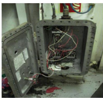
Improperly Modified & Maintained Certified Safe Junction Box
