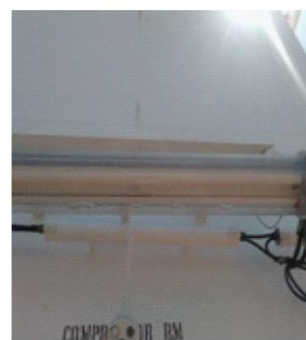
Standing Water in a Certified Safe Flameproof Light Enclosure Indicating Failed Ingress Protection
