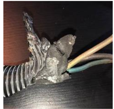
Fire spread to cable conduit
