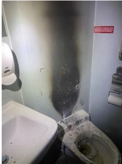
Showing damage to wall in bathroom
