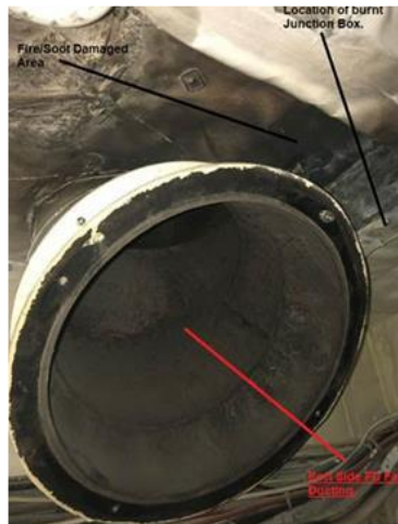
Port Side exhaust fan ducting
