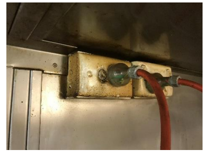
Fat residue accumulation on the power sockets
