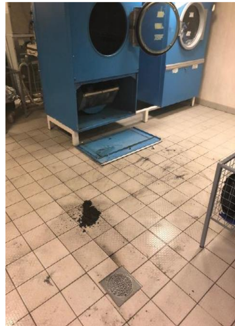
Laundry Room with tumble dryer in the background (Dust from smouldering laundry can be seen on the floor)
