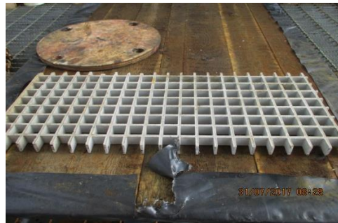
Piece of grating that dropped
