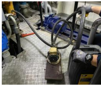
Pump rigged for procedurally correct transfer operation
