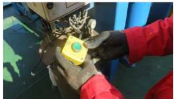
Remote control which failed
