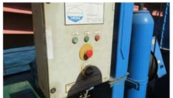
E-stop which failed to stop the winch
