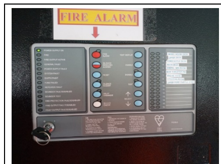
Disabled audible fire alarm
