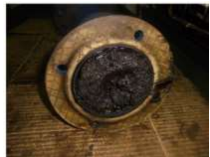
Completely blocked sludge discharge line
