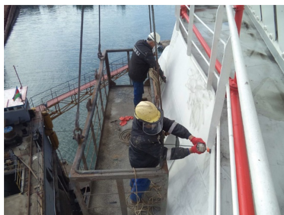
Working at height without a safety harness
