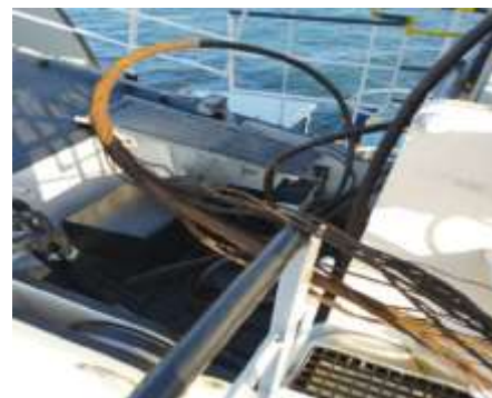
Parted wire frayed end
