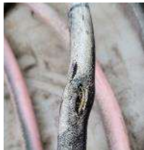
Damaged section of three-phase cable
