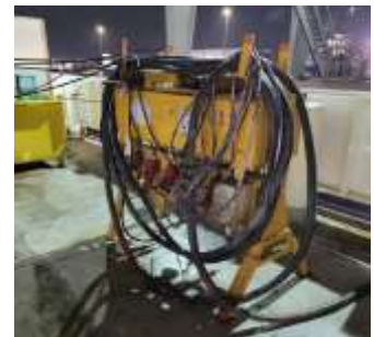
Shipyard electrical distribution box
