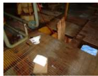
Post-Incident Photograph of hazardous grating section
