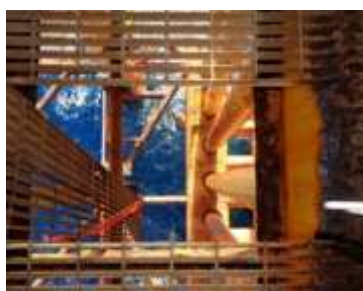
Post-Incident photograph of hazardous grating section suspended in open hole
