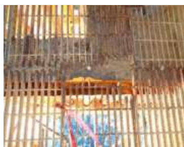
Pre-Incident photograph of hazardous grating section
