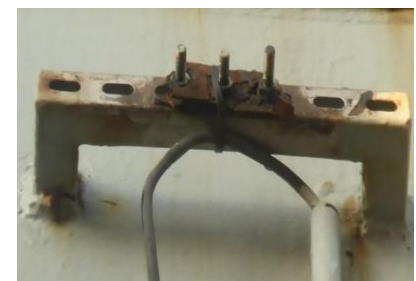
Flood light mounting frame
