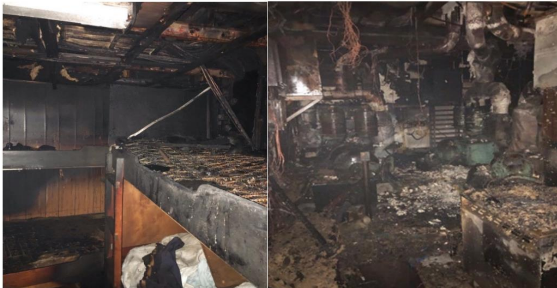
Fire damage to living quarters (left) and generator room (right). (Source: Coast Guard)
