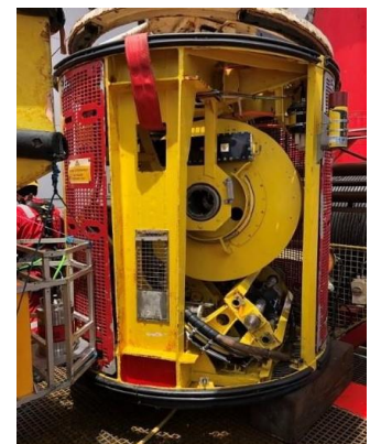
Showing a TMS door missing
