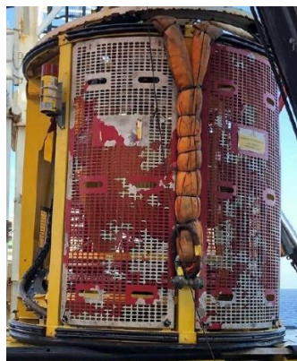
Showing a TMS door in place
