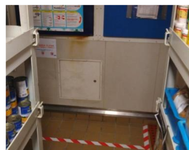
the switchboard, clear of flammable material with 'keep clear' zone marking in place.
