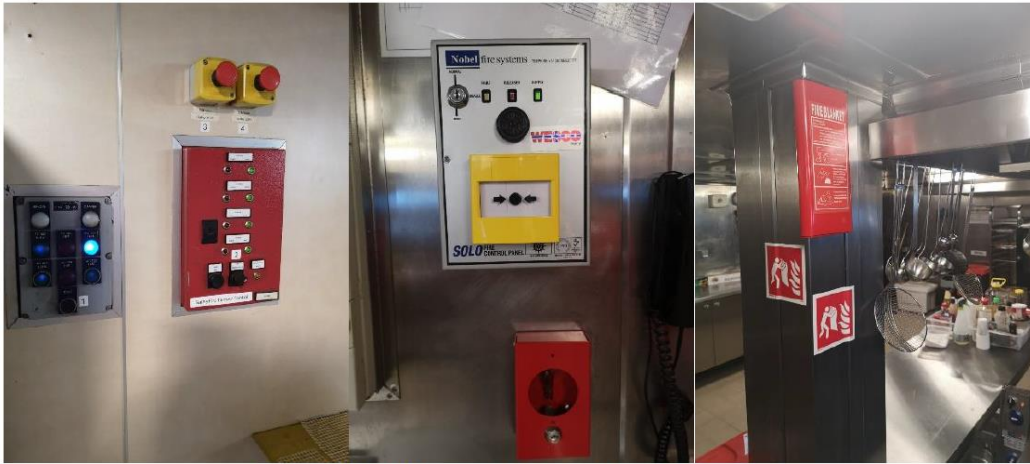
Galley firefighting systems and emergency stops
