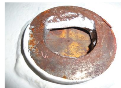
Portion of pin remaining on door
