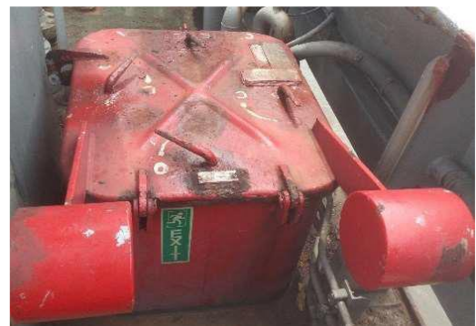
Escape hatch rusted closed
