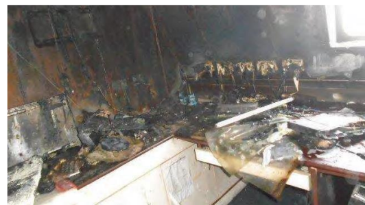
Burnt out day room of cabin
