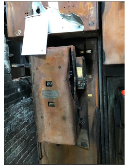
Photograph of the HV circuit breaker taken after the catastrophic failure, which resulted in fire and explosion within the substation.
