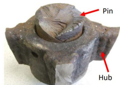
Accommodation ladder connection pin with severe corrosion over the pin's fracture surface & sidewall and on the surface of the hub.
