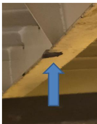
Impact damage from flying chain directly above
