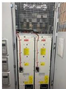
Open cabinet with fuses on top
