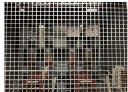
Fuses behind protective mesh
