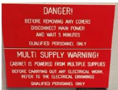
Signage on cabinet door
