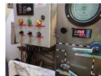
Exhaust valve open, visual and audible alarm
