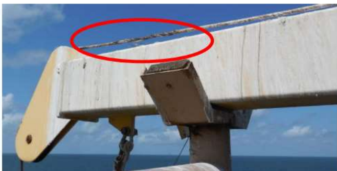
Figure 1 – Corroded crane cable
